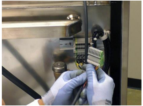
24. Locate the end of the power cable for the PVF.
